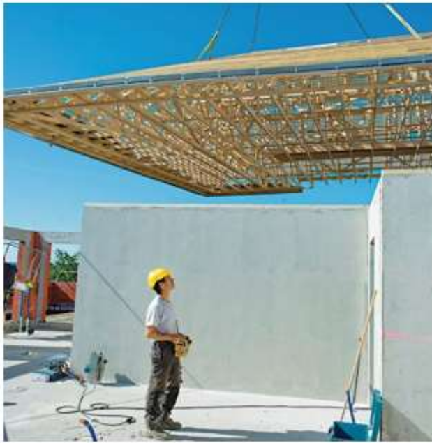
Installation of a roof truss on a multi-residential building, assembled on the ground, then mounted with a remote-control crane.
