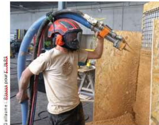
Projection of a coating comprising a mix of hemp fibres, dry earth and a slip (semi-dry process) to design an insulating panel.
