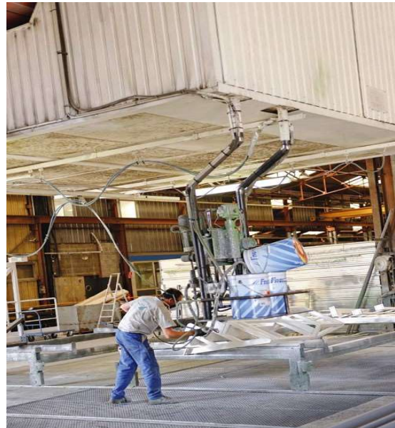
A mobile extraction system for paint, outside of a booth
