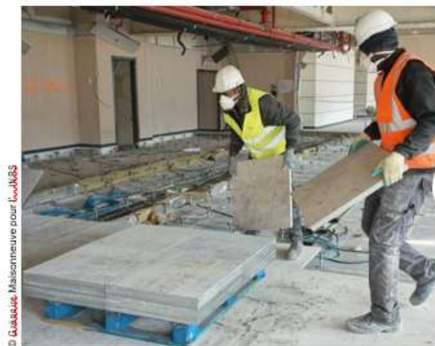
Workers manually remove a raised floor in view of its reuse for a new construction.
